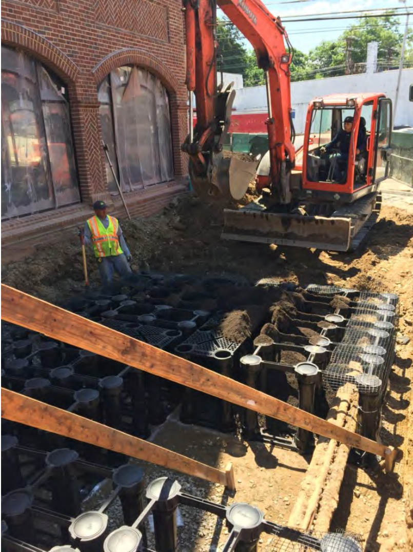
Taken by Al Key on June 21, 2016. Silva Cell installation with soil added via bucket loader, not swept in.
